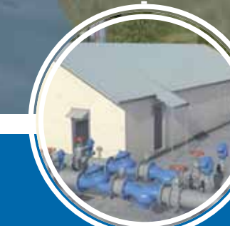
PRESSURE REDUCING SYSTEM
