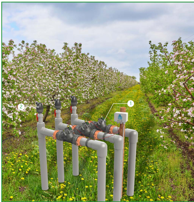
[1] BERMAD Model IR-11T opens & closed upon to electric command [2] Combination Air Valve
